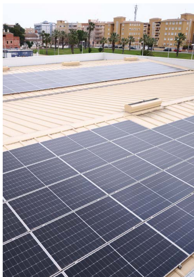
Solar panels at the Moncofa Consum
